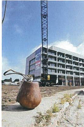
A 5,000-pound wrecking ball sits ready for work as the shell of what used to be the March Air Force Base Hospital stands for the final time in the background. Demolition began on the March hospital building during a deconstruction ceremony Tuesday, March 22, to make way for the $3.3 billion March LifeCare campus. (Photo courtesy of Matthew Smith)
